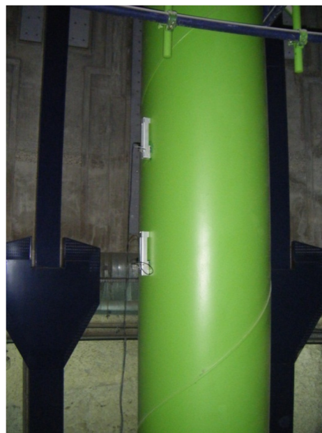
Check of a worn water discharge pump
